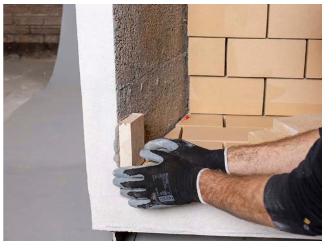
Once the bottom and rear firebricks are in place, fasten the side bricks in position using the firebrick mortar. Use a tile spacer to keep an 8mm gap.
