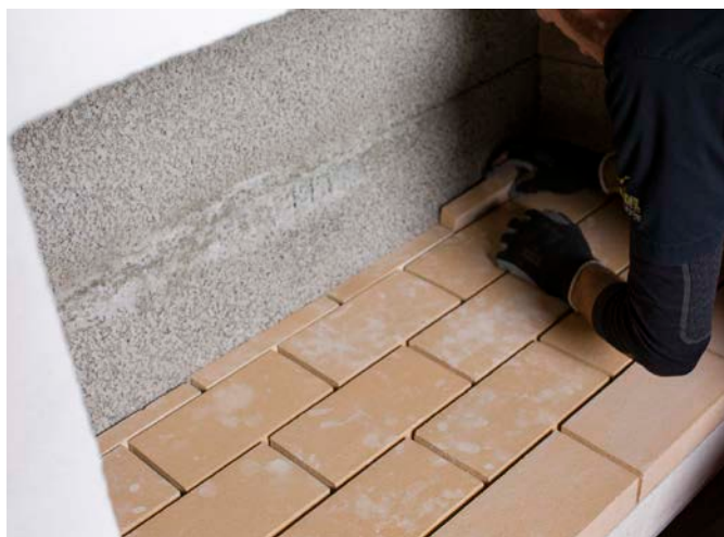
Complete the bottom layer of firebricks, then fasten the rear firebricks in place using the firebrick mortar. Use a tile spacer to keep an 8mm gap.
