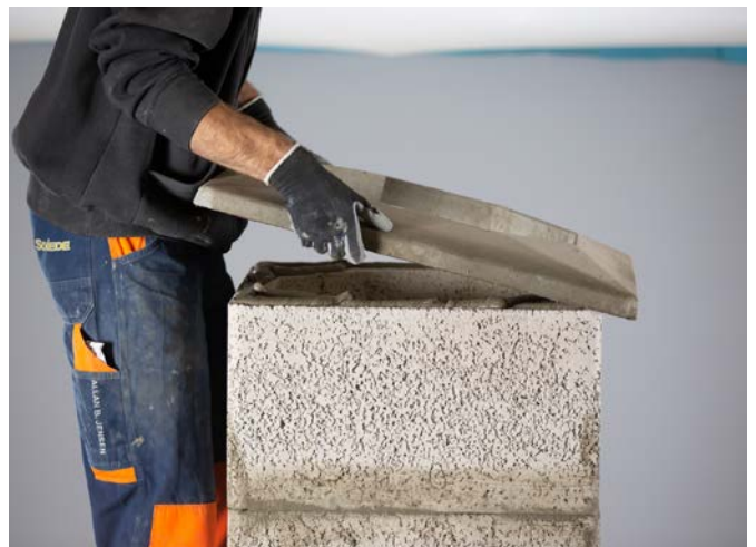
If the capping is purchased, then glue the top of the final chimney block as per previous instructions and then place the capping on top.
