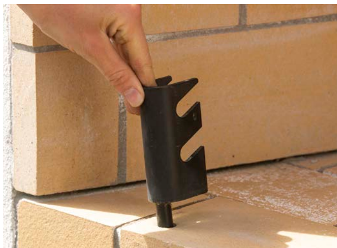
Drill 2 x 12mm diameter holes in the front row of the firebricks. Push log retainer holders in place.
