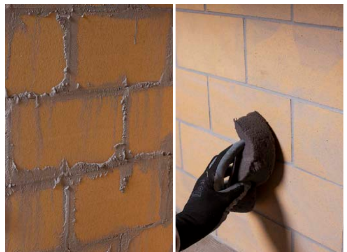
Use the mortar mix to point up the joints between the firebricks once they are all in position. Clean off excess mortar.
