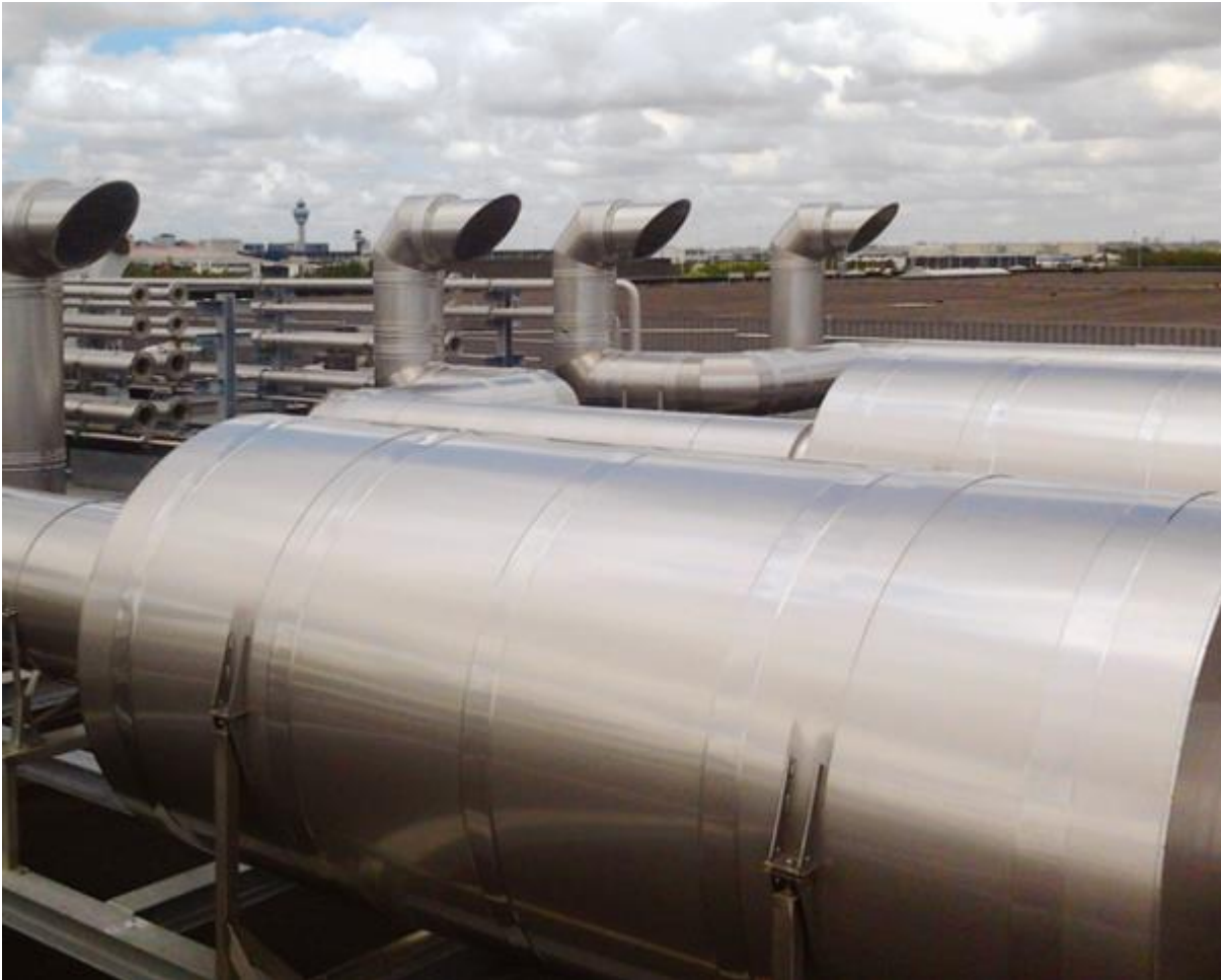
A range of silencers installed on a Metaloterm Flue System
